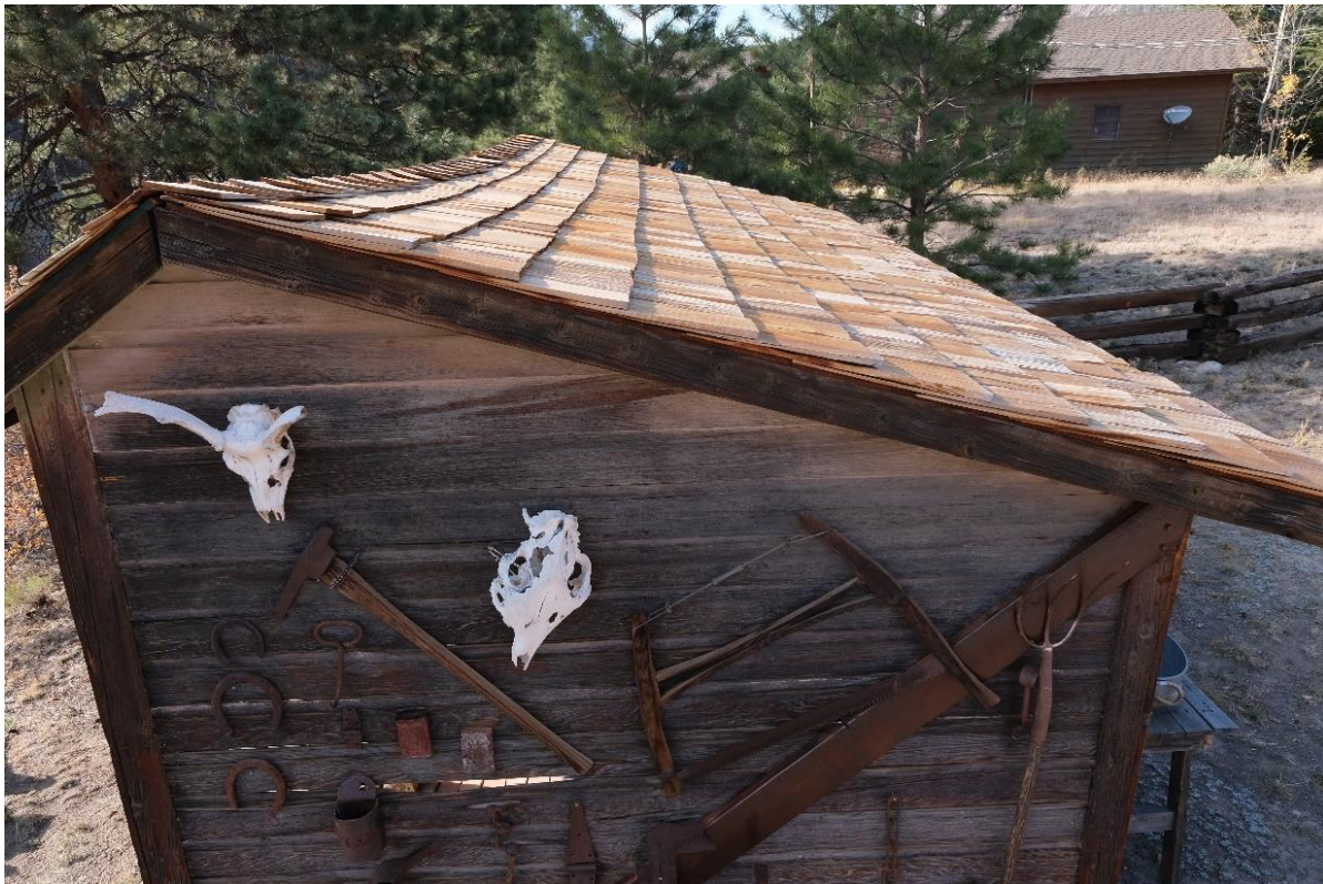
Figure 20. View of the exterior top of the 'Waiting House,' depicting the roof's pitch with the new shingles, replaced in 2019 (eastern aspect).
