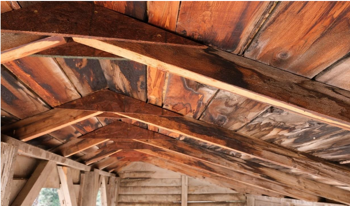
Figure 19. Interior view of the 'shed gable' roof (eastern aspect). The triangular supports added by Kim Marvel in 2019 are shown along the eave of the roof.
