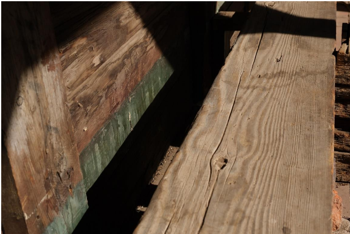
Figure 23. Original green paint behind the bench on the northern-most interior wall. Evidence of white paint on the planks above are also observed (western aspect).
