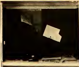
A wall partially ripped.
