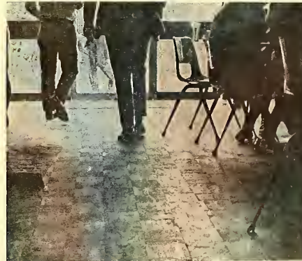
IS THIS A MONUMENT to CC history? The first floor of its kind in the state of Colorado brightens up our Hub. (But it leaks oil.)
