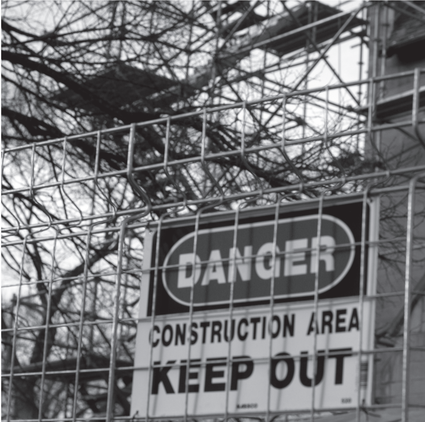
Fencing surrounds the construction site at Shove Chapel where workers are restoring a section that was struck by lightning in August
