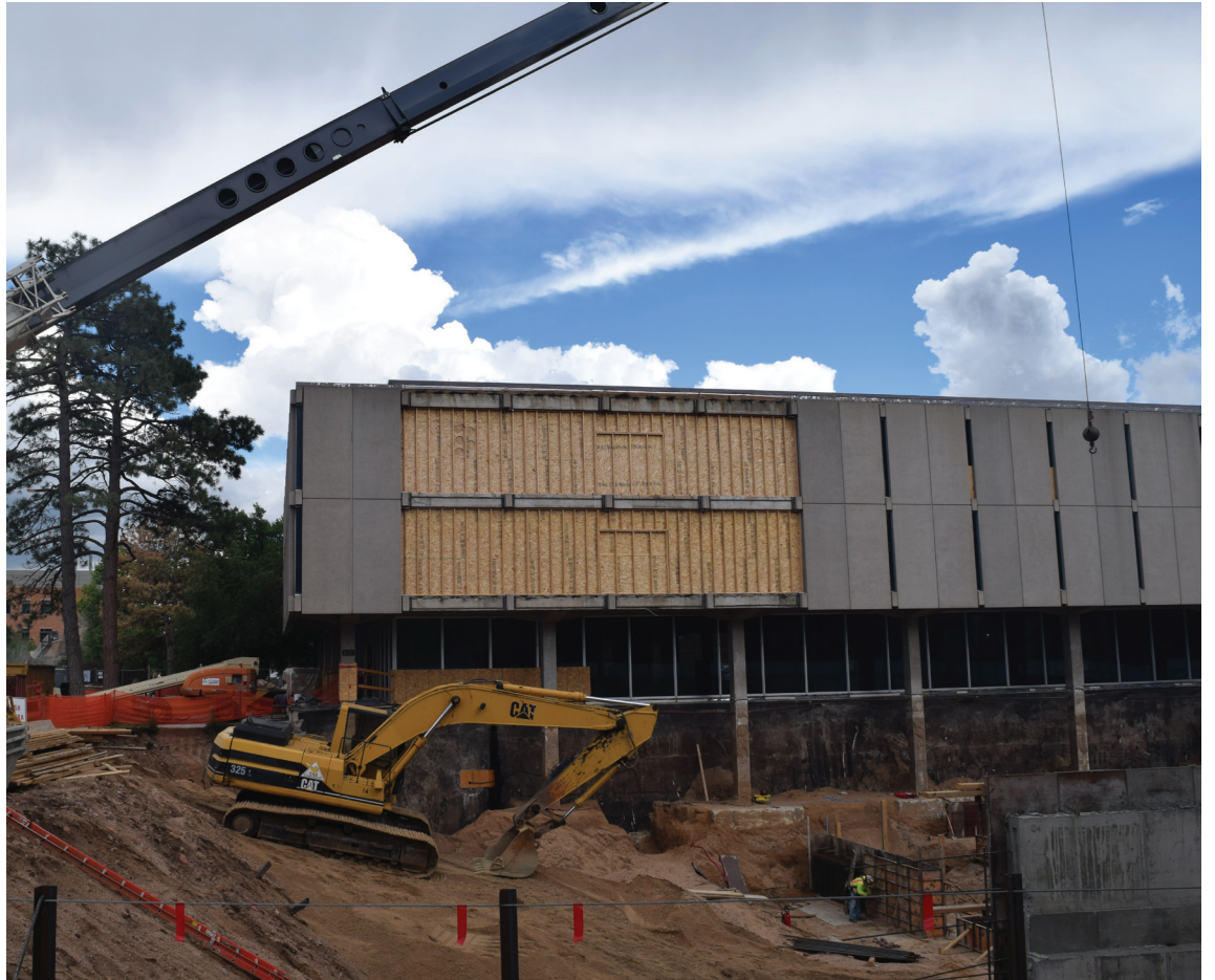
PHOTO BY NATE MONGA. Tutt is gutted in the early stages of a large renovation that will be completed by the beginning of next fall semester.
